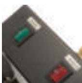
separate power and light switches
